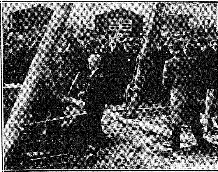
Here is James G. McDonald, League of Nations High Commissioner, driving the first pile as the work of developing the "Werkdorp Nieuwsluis" colony for exiles from Hitlerite Germany began. The colony is situated on land reclaimed from the Zuyder Zee.
